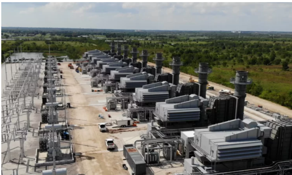
The Tpoaz Generating Station near Houston, Texas, is similar to the facility that ProEnergy is proposing to build near Centre Village in the Tantramar area, according to ProEnergy. Source: ProEnergy.
