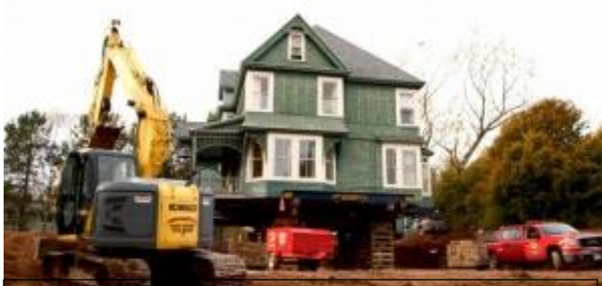
Figure 6 – 2013 – the former Mt A satellite residence, Cuthbertson house , was sold and moved to a new location by purchaser Jim Throop, to be restored and improved, then rented to off-campus students.
